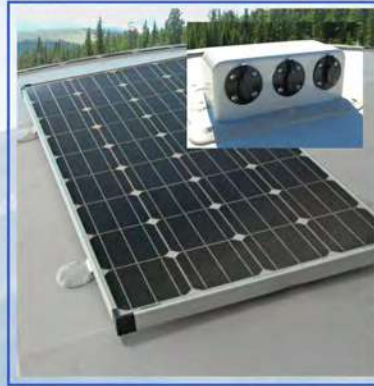
170 Watt Roof Mounted Solar Panel
