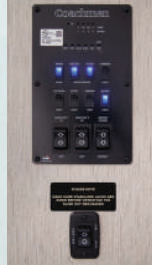
Centralized control panel
